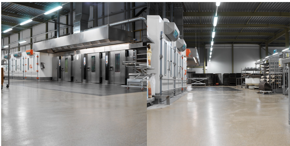
Industrial mortar in bakery (Primer 300 gr/m 2 , 14 kg UniQuartz TK 11 with binder 15% of the filler, Topcoat 200 gr/ m 2 EP High Gloss Thix)
